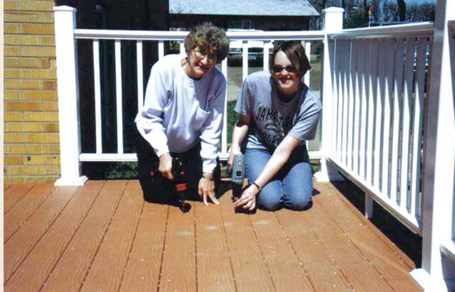
Dakota Hills Assisted Living Home in Elgin, N. Dak., has a beautiful new deck due to the efforts of Mott Branch 79, Grant County FFA, and Girl Scout Troop Phelan 1100. Due to frost concerns, landscaping around the deck took place on a later date.
