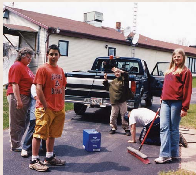
Northwoods Branch 925 and WRVM Christian Radio Station volunteers put in new pavement for their JOIN HANDS DAY project at the nonprofit radio station.
